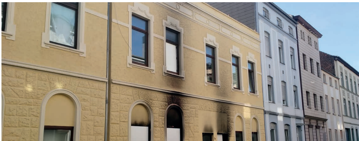
Abb. 3: Problemimmobilie in Düren
